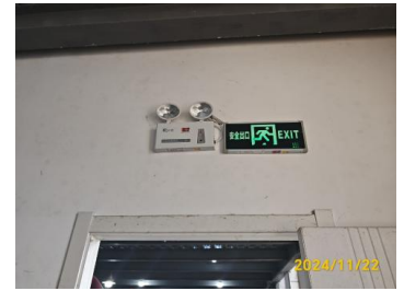
Emergency light and exit sign.jpg
